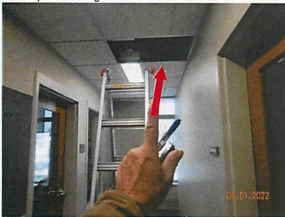
39. Data Logger #8 is placed above the suspended ceiling in the south return air plenum
