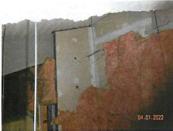
31. View of displaced/missing insulation on unconditioned side of the east mezzanine wall.
