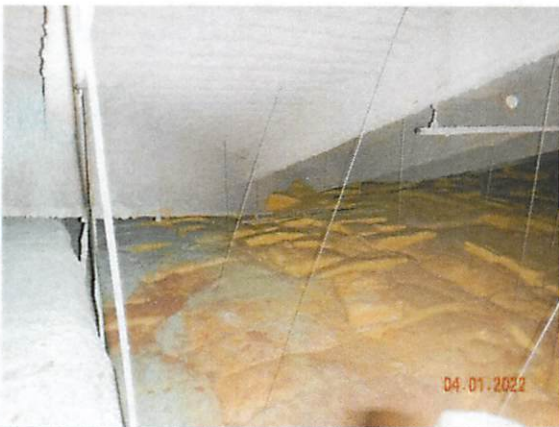
27. View of the south valley of the west roof within the attic space south of the mezzanine. Soffit vent tubes were not visible between rafter to the right of the valley.
