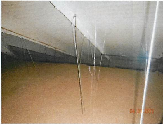
15. Typical view of the cellulose insulation in attic above the 3 rd floor mezzanine. Air flow space between insulation and roof appears adequate.
