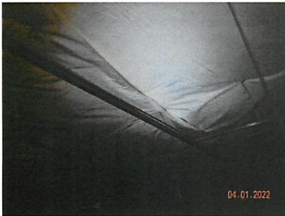
47. View of lapped but unsealed plenum air/vapor barrier.
