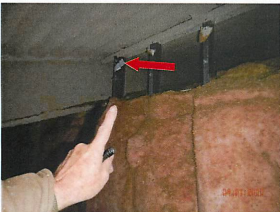
29. View of Data Logger #5 placed towards the upper portion of the unconditioned side of the east 3 rd floor mezzanine wall. Note, space between wall and roof deck appears to allow for adequate air flow to mezzanine attic.
