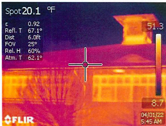
5. Partial IR image of the east roof. Note, temperature at the eave and field of the roof are similar.
