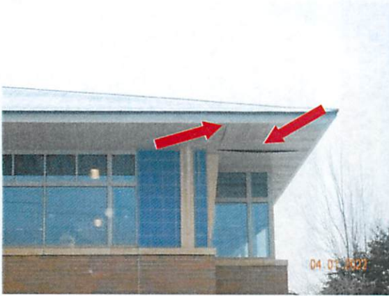
13. Displaced soffit panels at northwest corner.
