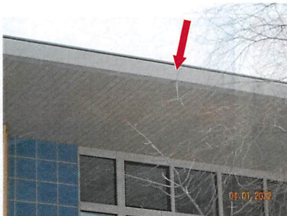
11. Ice icicle at gutter seam along east roof eave.
