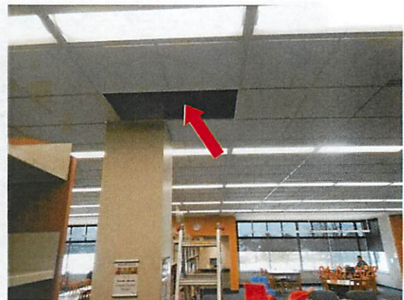
40. Data Logger #9 is placed above the suspended ceiling in the north return air plenum.
