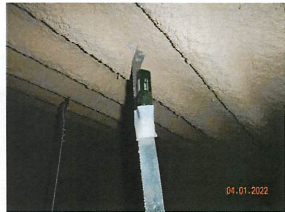
22. View of Data Logger #4 in the 2 nd floor attic space south the 3 rd floor mezzanine.
