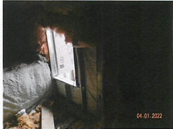
32. View of displaced/missing insulation on unconditioned side of the east mezzanine wall.
