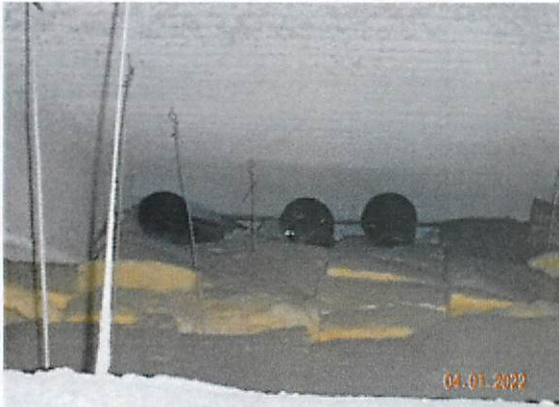
25. View of 10" to 12" metal tubes that have been installed at some of the soffits to provide air flow. West attic/soffit interface of the attic space south of the mezzanine shown.
