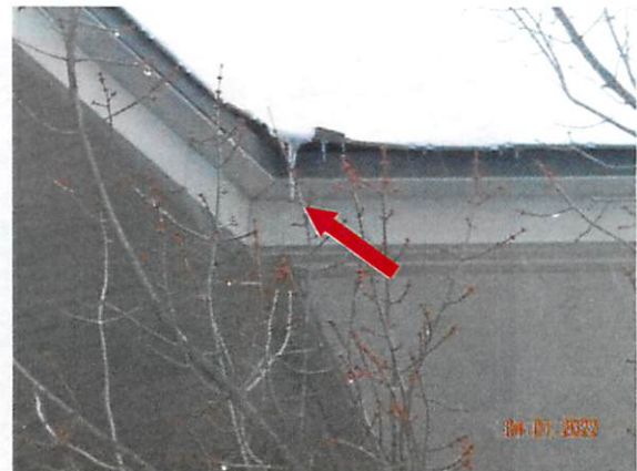
12. Ice at valley along west roof eave.
