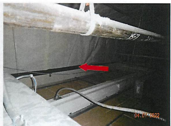
42. Interface lap joints appear to be sealed at some locations in the south plenum.
