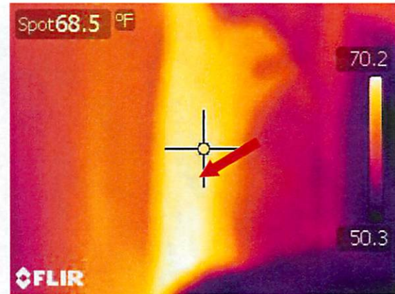
24. IR image of Photo 23. Bright yellow/orange is attic access door and heat-wash.
