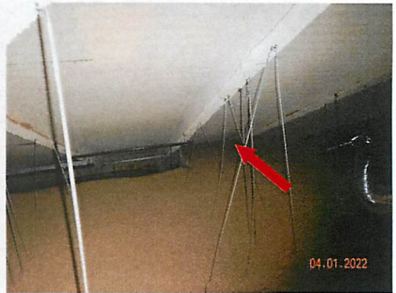
16. Typical view of the cellulose insulation in attic above the 3 rd floor mezzanine. Air flow space between insulation and roof appears adequate. Arrow shows location towards south end of east perimeter where air flow space is reduced.
