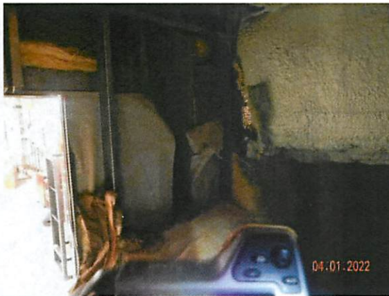
23. View of missing insulation and incomplete/open plastic air/vapor barrier adjacent to the south mezzanine access panel to the attic space.
