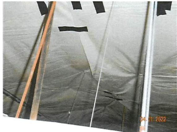
48. Another view of lapped but unsealed plenum air/vapor barrier.
