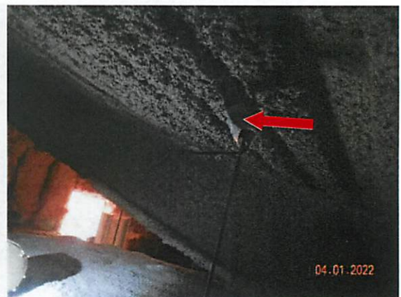
30. View of Data Logger #6 in the 2 nd floor attic space east of the 3 rd floor mezzanine.
