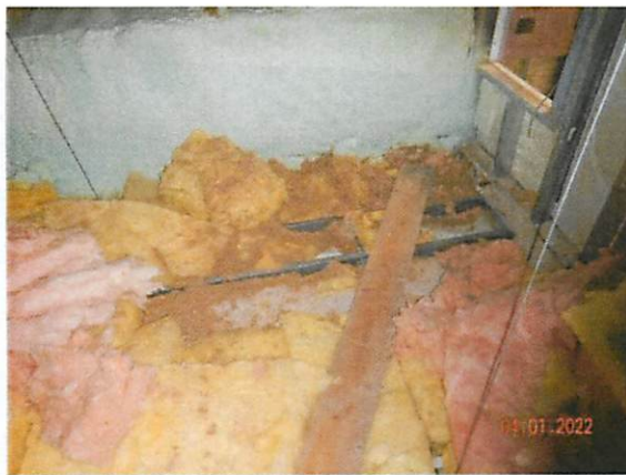
33. Displaced and missing insulation at 2 nd floor plenum ceiling in the attic space east of the 3 rd floor mezzanine.
