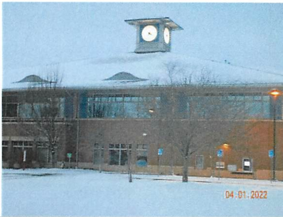
3. Partial view of the east roof. Reference Photo #5 for IR image.
