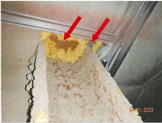
45. Cardboard and spray polyurethane foam (SPF) has been installed at the plenum column penetration where Logger #22 was placed in the north plenum.
