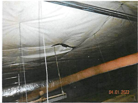
46. View of taped air/vapor barrier seam in the north plenum that has failed adhesion.
